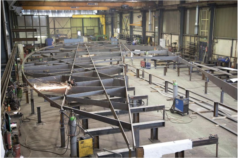
Figure 3.13 The roof was prefabricated in the workshop, then divided into seven transportable segments and assembled on the ground immediately next to the final location. © Ingo Schrader Architekt BDA.
