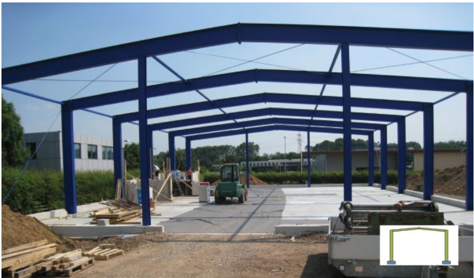
Figure 6.4 Single-storey building with a steel frame, symbols for steel frame in grade S 355. © Kerschgens Stahl & Mehr GmbH.
