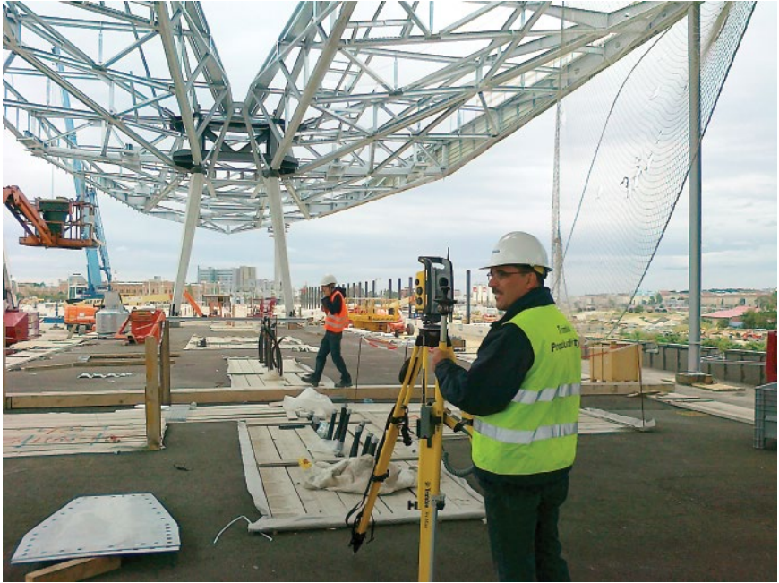
Figure 3.10 With the help of the Trimble total station and the data from the BIM model, the roof elements were precisely positioned. © Trimble.
